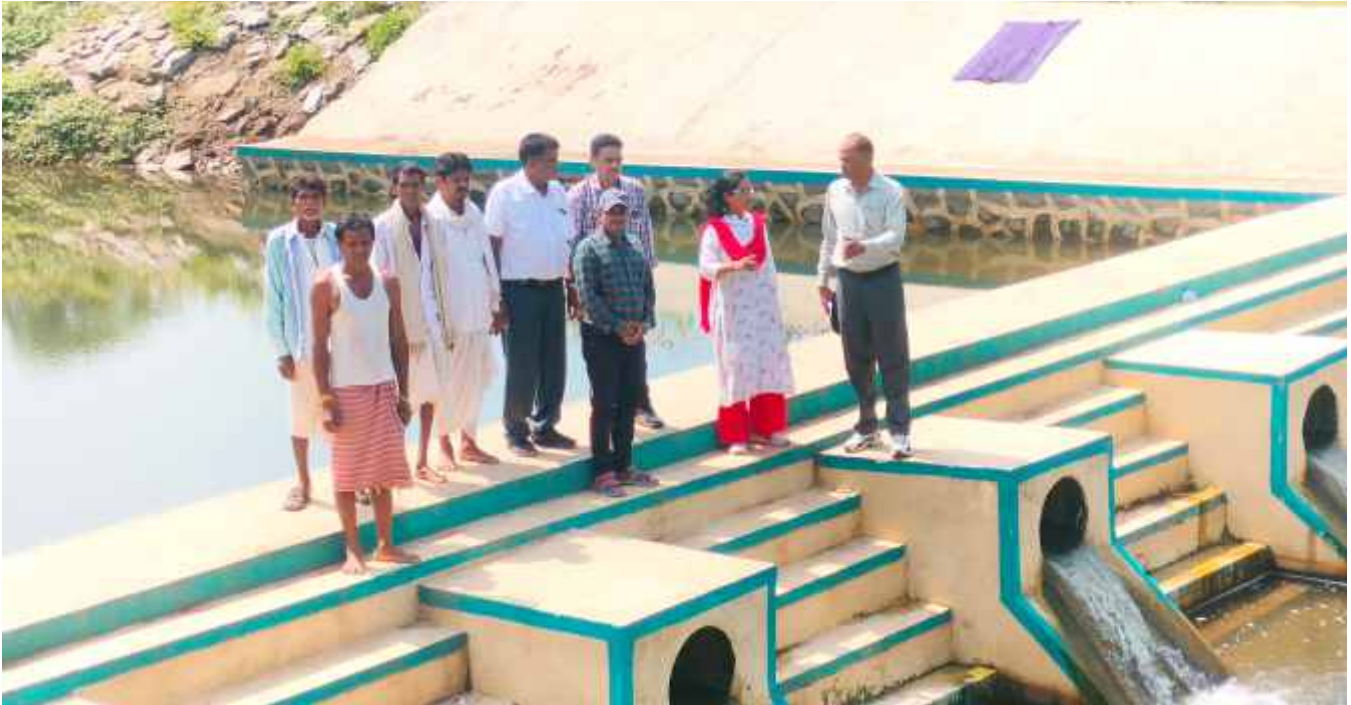
Shri Dalip Singh, Joint Director, Agriculture, Banswara visited Padlamokha check dam built under RKVY project in Banswara district.
