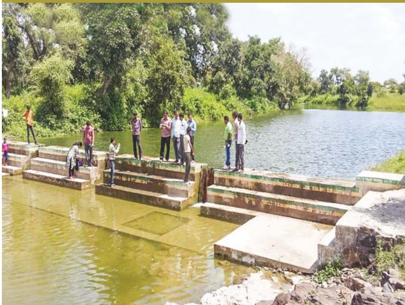
Small water harvesting structure at village Kotdi, tehsil Sitamau, district Mandsaur, Madhya Pradesh under IWMP-I.
